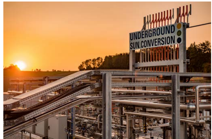
RAG-Anlage in Pilsbach/Oberösterreich, Fotos: RAG Austria AG/Karin Lohberger Photography
