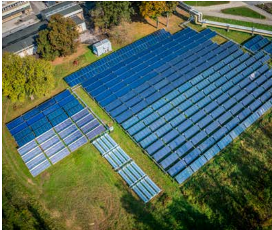
Collector test of various collector types with 3,123 m 2 for solar district heating feed-in at the district heating plant Puchstrasse in Graz, Austria; Photo: S.O.L.I.D. GmbH
