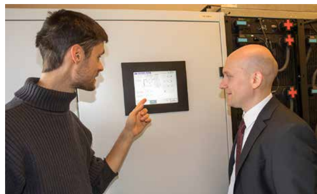
Heimschuh's storage system, all photos above: Energie Steiermark/icon
