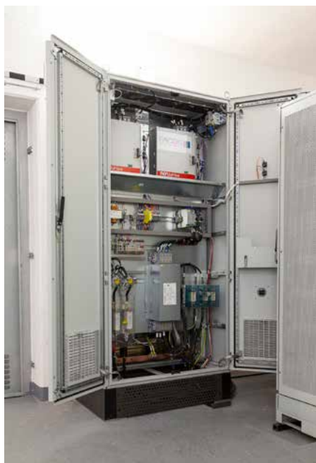
FACDS inverter, Photo: Wiener Netze GmbH
